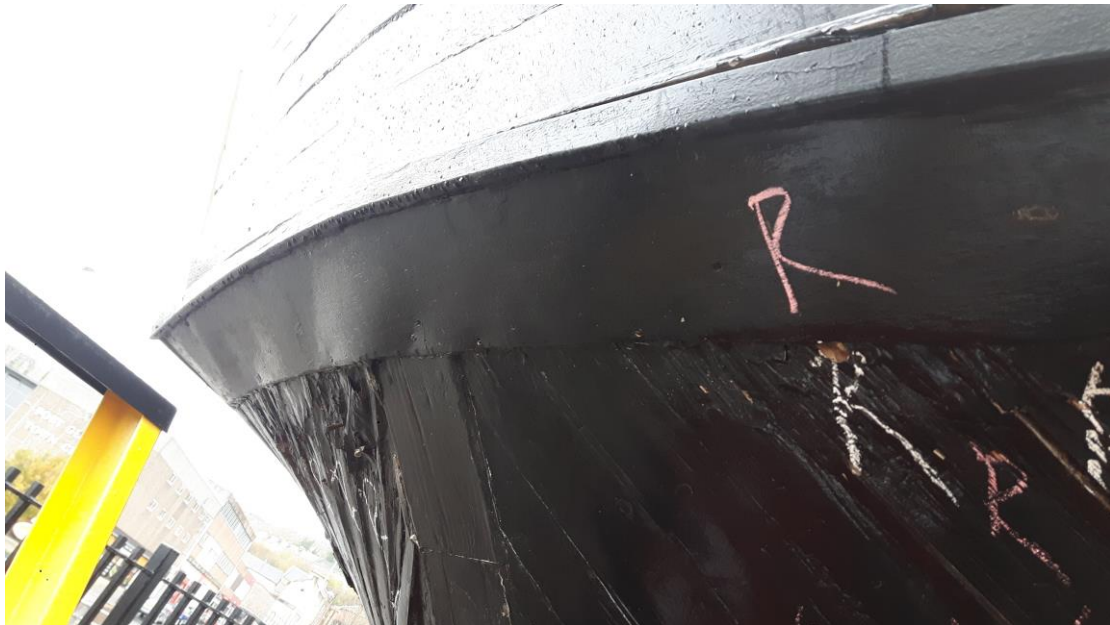
Typical coatings and plywood strip to keep planking in place in the stern
