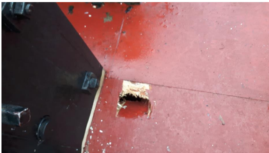
Rotten ply wood deck forward.
