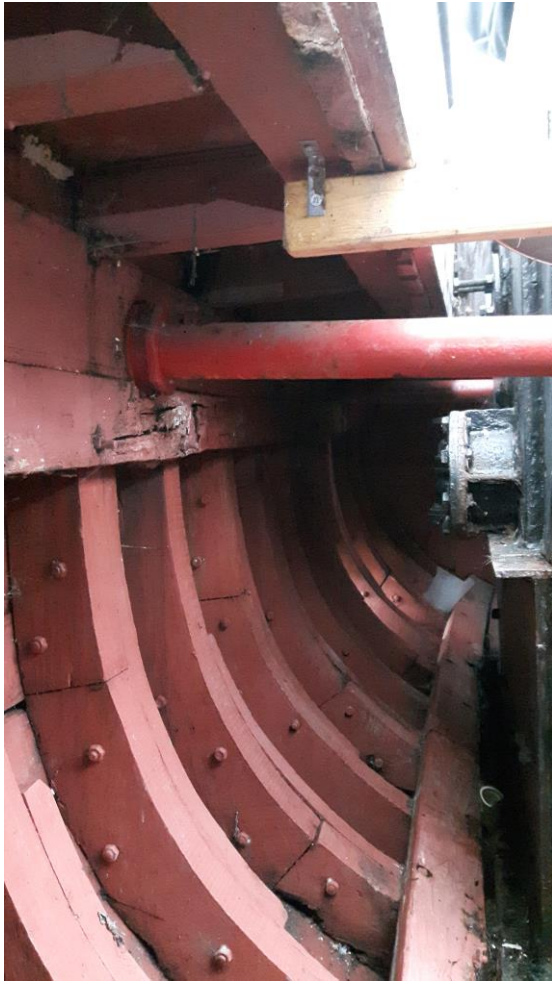
Framing in the engine room, rotten bilge stringer, rotten beam shelf, rotten beam shelf stringer
